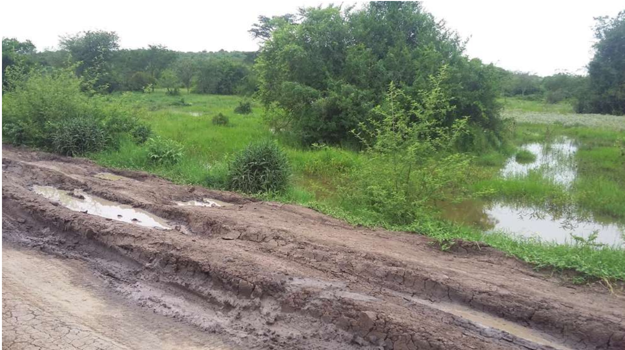
Plate 1: Flooding hotspot along the road in Kaliiro Sub-county
